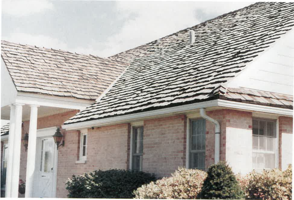
This gable roof shows excellent design and construction. Notice the valley flashing and complete gutter system.
