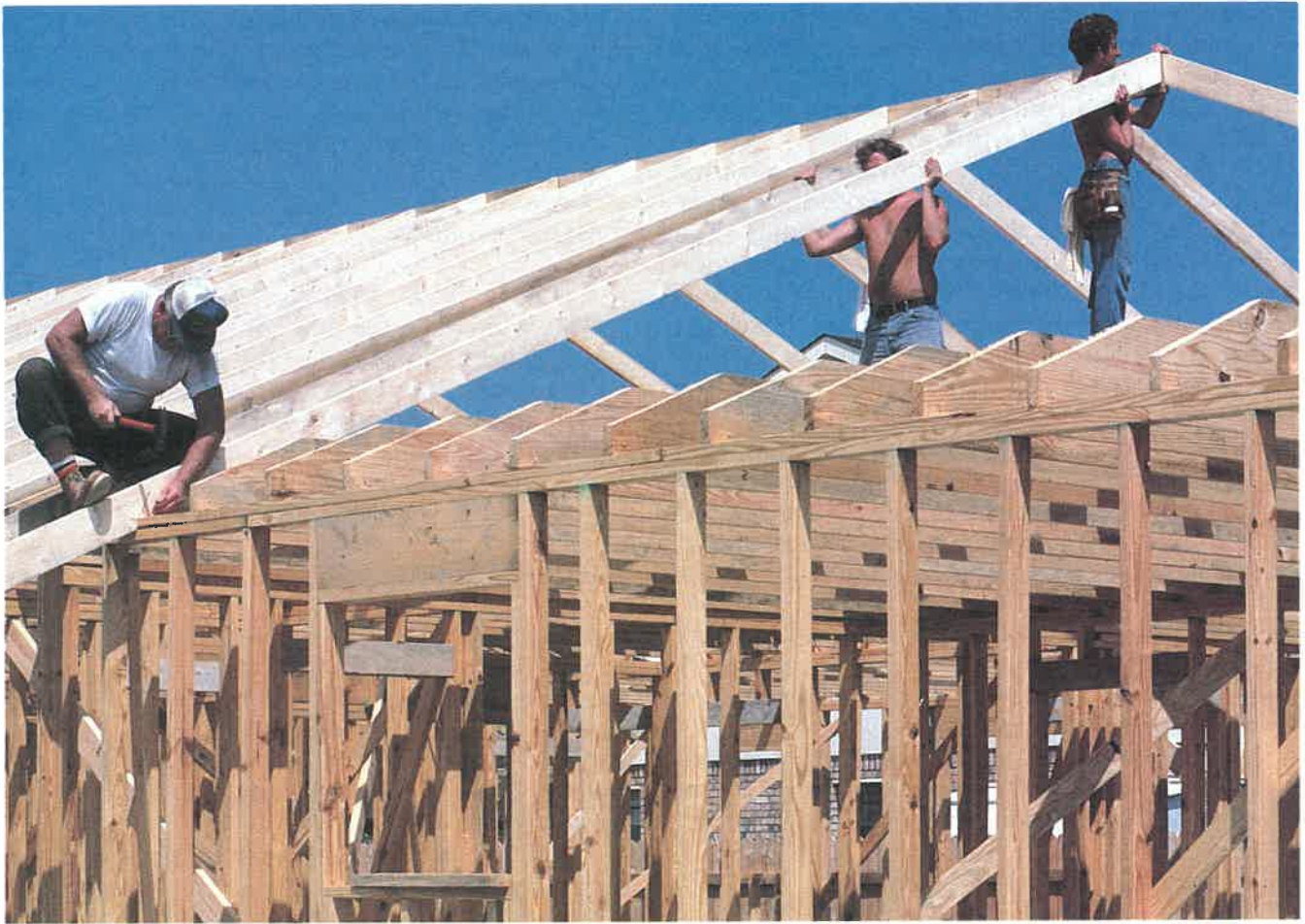
Fig. 28-10. Installing common rafters. Be sure bird's-mouth is pushed tightly against the plate. (Southern Forest Products Association)
