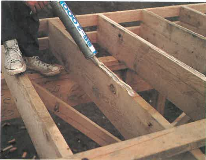
Fig. 27-34. Applying adhesive for a glued floor system. A 1/4 in. wide band of glue applied to the top of the joist is sufficient. Two beads are applied where panels butt. (American Plywood Association)
