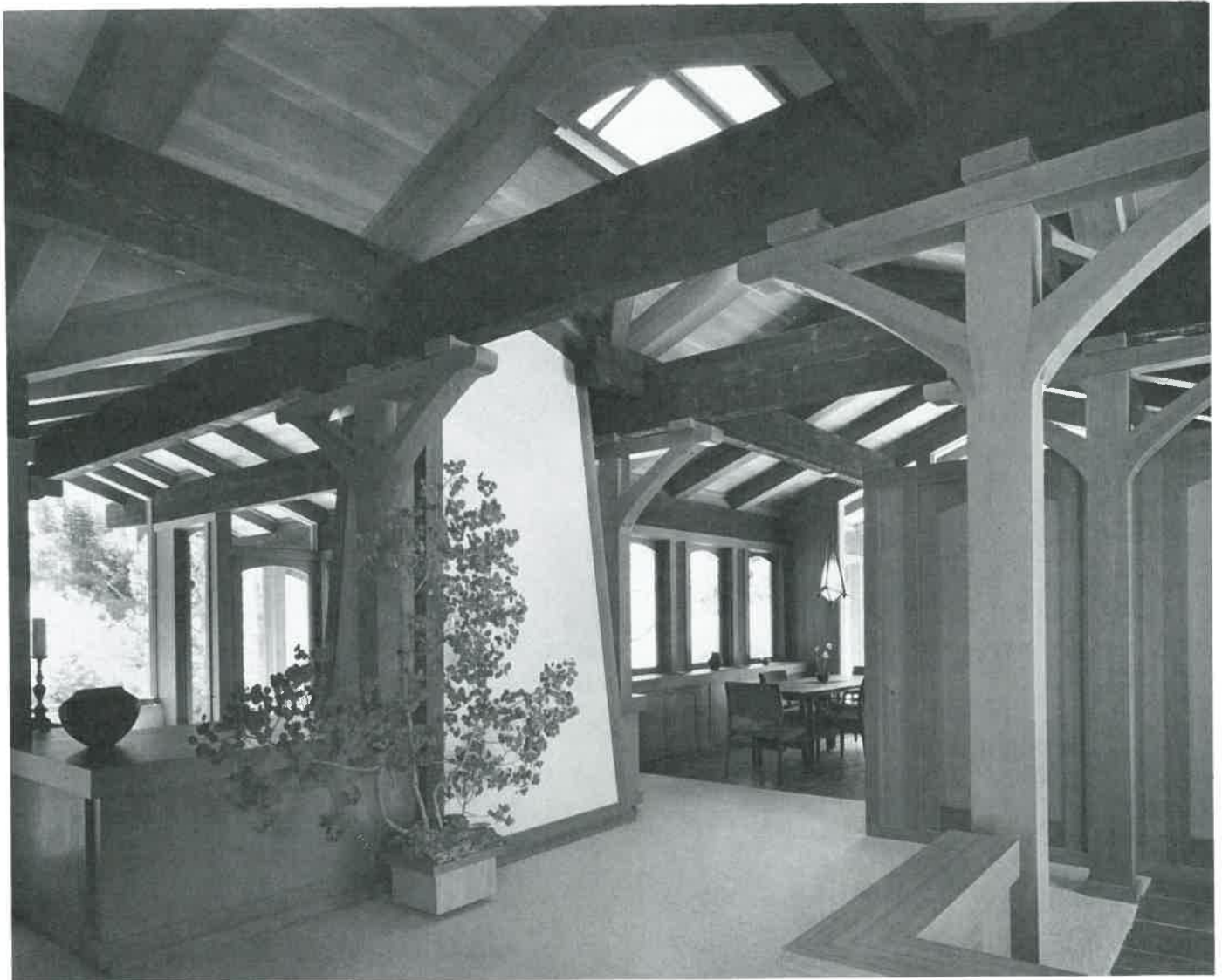
Fig. 31-3. An example of post-and-beam construction in a modern home. (California Redwood Association)
