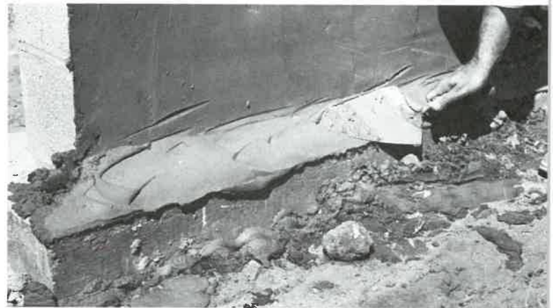
Fig. 26-32. A cove of mortar is formed over the footing to prevent water from entering. (Portland Cement Association)
