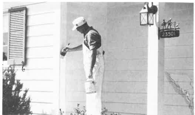
Fig. 12-34. Exterior latex (water-base) paint being applied to exterior surface. This paint has high resistance to blistering and peeling. (Sherwin-Williams Co.)
