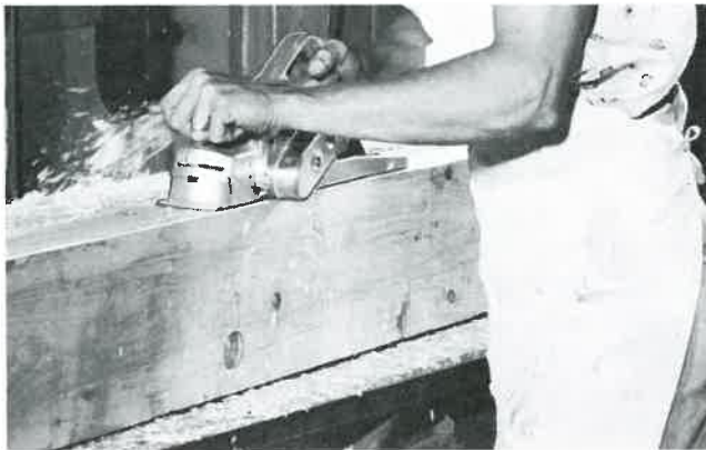
Fig. 13-23. Using a portable electric plane to surface a large beam. (Skil Corp.)
