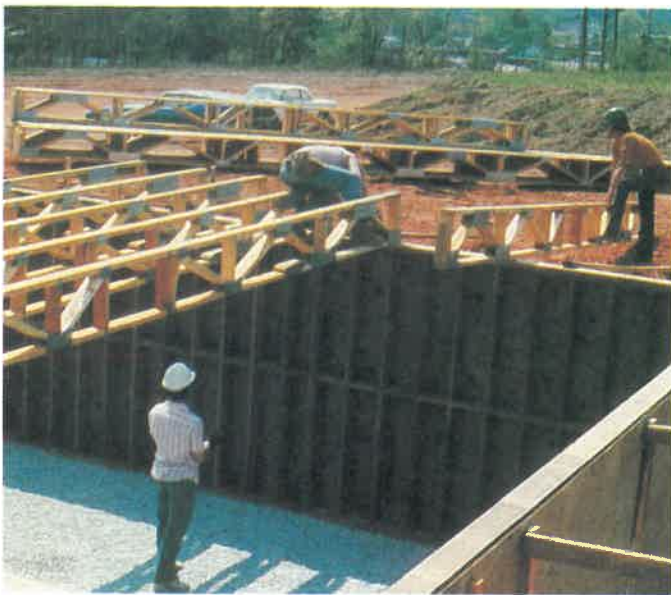
Fig. 26-40. Truss joists being installed over wood foundation. Use of 10d nails is recommended so inward pressure on wall is transferred to the floor system. (Osmose)
