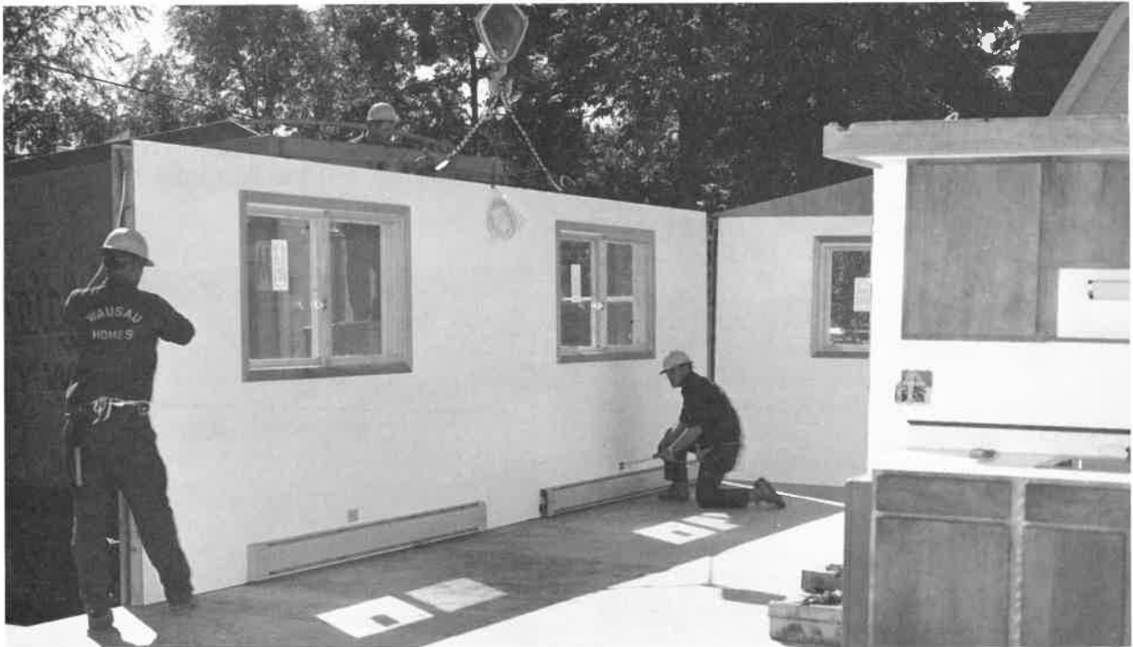
Fig. 31-18. A prefabricated wall panel is lifted into place. Notice that the electrical outlets, heating units, trim and wall finish have already been applied.
