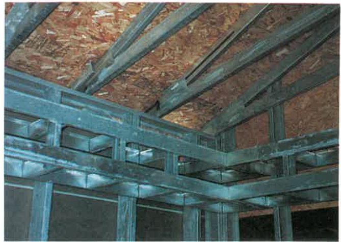
Fig. 27-64. Interior of metal framed residence showing portion of kitchen soffit from which cabinets will be hung.
