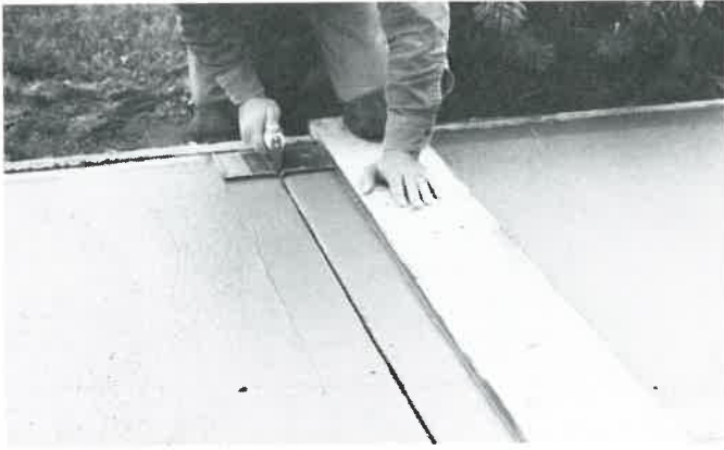
Fig. 26-37. Jointing a slab helps control any cracking due to shrinkage caused by dryness or temperature change. (Portland Cement Association)
