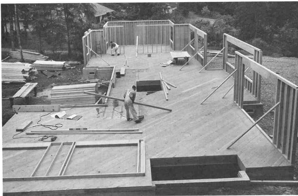
Fig. 27-49. Wall frames are assembled on the floor and then raised into position. (National Forest Products Association)
