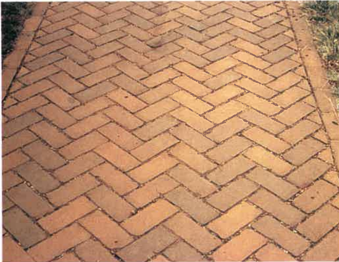
Fig. 26-38. Brick paving can be installed either as a rigid or flexible system.
