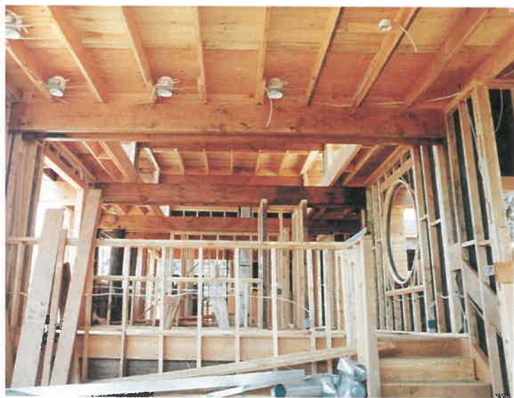
Fig. 30-1. A residence during the rough-in phase. Several lighting fixtures and receptacles are in place and duct work is in process. Rough heating, plumbing, and electrical are installed before the insulation and interior wall finish is applied.
