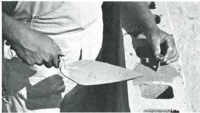
Fig. 26-28. Anchor bolts and straps are installed about the same way. Top. Anchor strap is embedded in the next-to-top block. Bottom. Embedding an anchor bolt in concrete or mortar.
