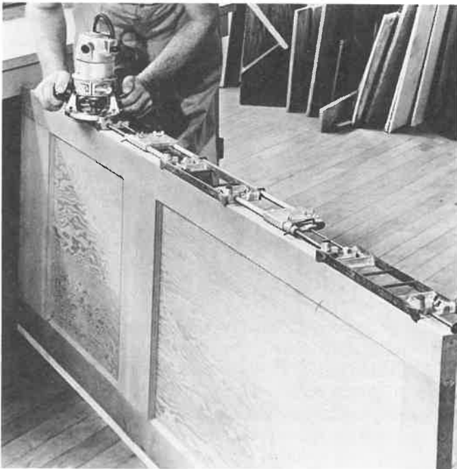
Fig. 18-21. Using a special template to cut the gain for passage door hinges. This template will also be used on the door jamb.
