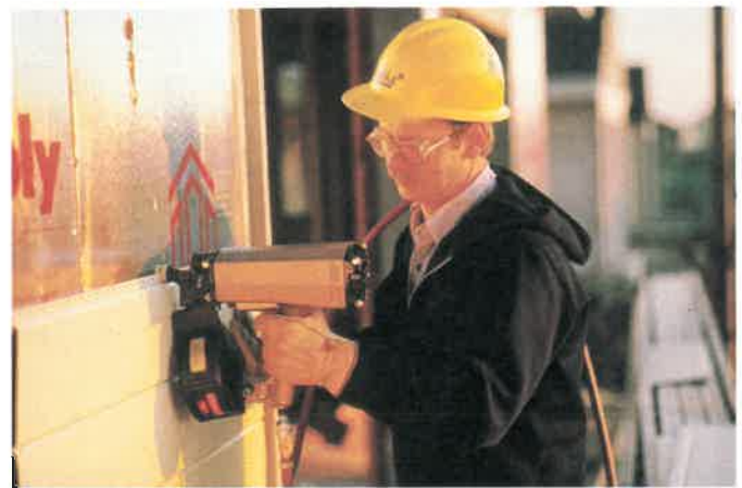
Fig. 29-31. Installing an aluminum siding panel. Lower edge interlocks with previously applied course. (Alcoa Building Products)
