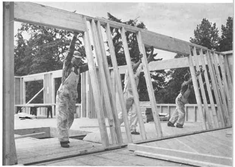
Fig. 27-51. Raising a main bearing partition. Note that a section of the double plate has been used to splice the top plate.
