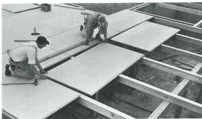
Fig. 31-7. Laying 1 1/8 in. plywood with tongue-and-groove edge joints on beams spaced 4 ft. O.C. (American Plywood Association)
