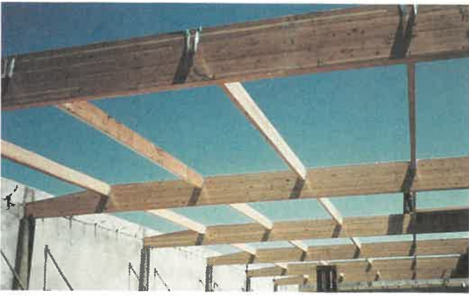
Fig. 23-21. Laminated beams provide a clear span of 48 ft. Purlins, spaced at 8 ft., will support 4 x 8 ft. prefabricated roof panels. Note the metal connections used to fasten the purlins to the beams. (Boise-Cascade Corp.)
