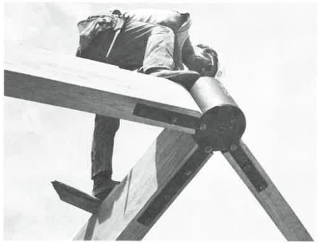
Fig. 23-22. Construction worker attaches beam brackets to steel drum. The drum serves as a hub for assembling major beams. (Koppers Co., Inc.)
