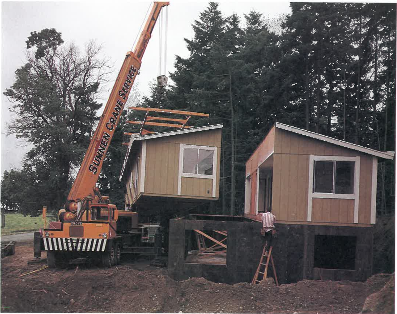
Sectionalized (modular) home being placed on its foundation. Each module is completely finished inside and out. (American Plywood Association)
