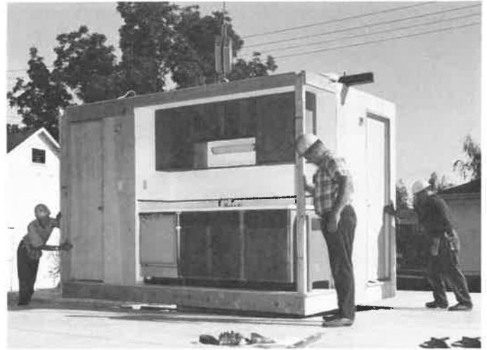
Fig. 31-19. This kitchen module is being lifted into place. Other walls of the house will be located around it. Note the dishwasher, sink, and lighting fixtures have been installed.
