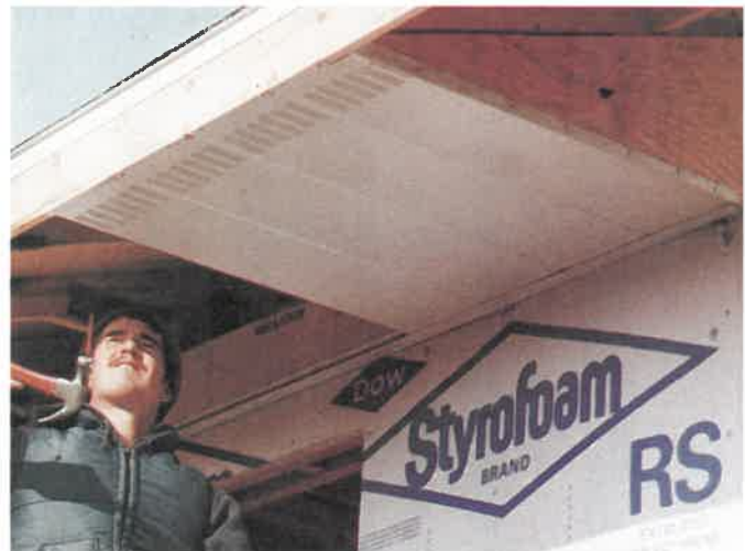
Fig. 29-25. Prefabricated metal soffit system being installed on a wide boxed cornice. Each panel is 9 in. wide.
