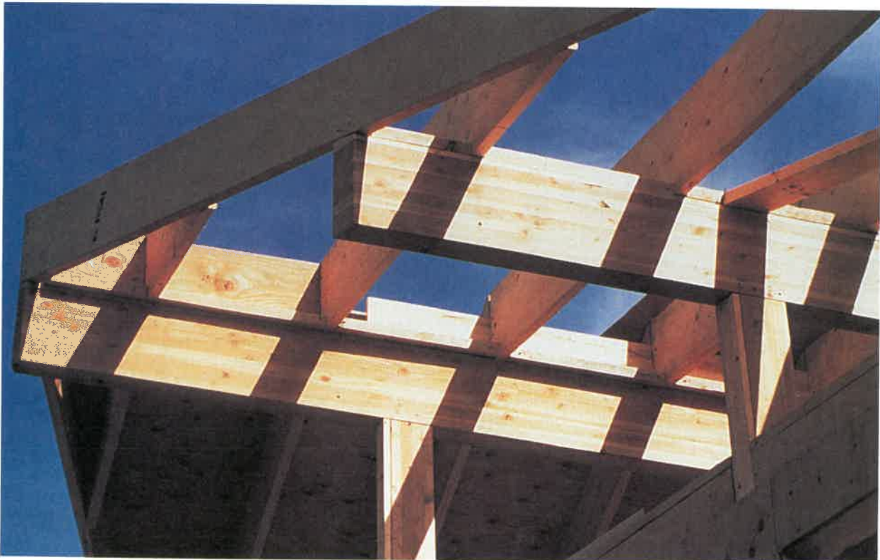
The roof structure of this residence is supported with glue laminated beams. (American Plywood Association)
