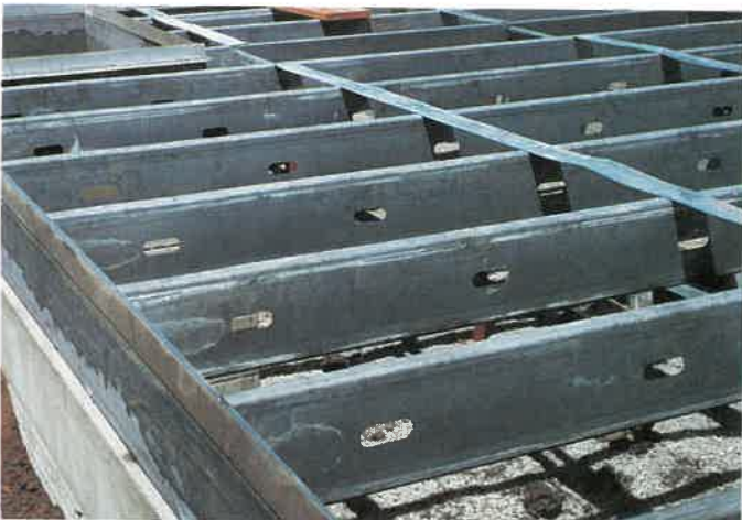
Fig. 27-35. These steel joists are attached to a steel header resting on the foundation. A plywood subfloor will be installed over the joists.
